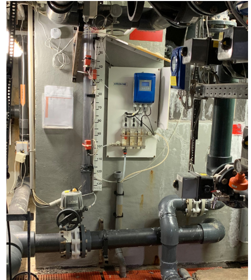
Bypass measurement for monitoring free chlorine in a thermal bath pool
